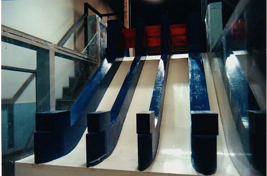
1) Looking upstream from the stilling basin to the Skeleton Bay Surface Bypass spillway crest and piers. (R15-15)
